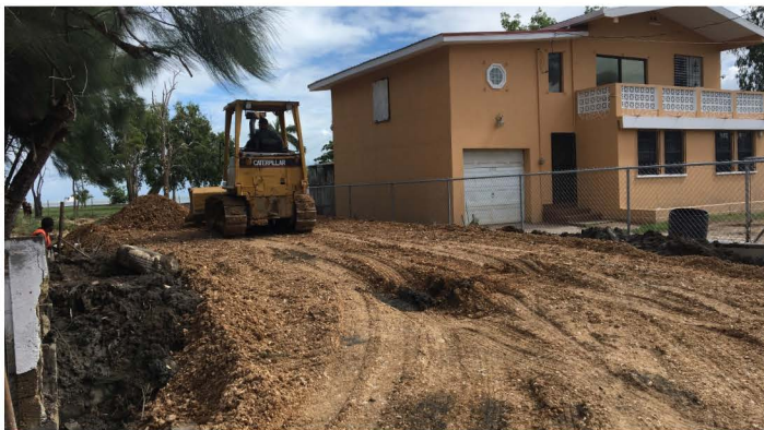
Not only did Cisco Construction Ltd. donate the fill but also the machinery to spread the fill on the lot
